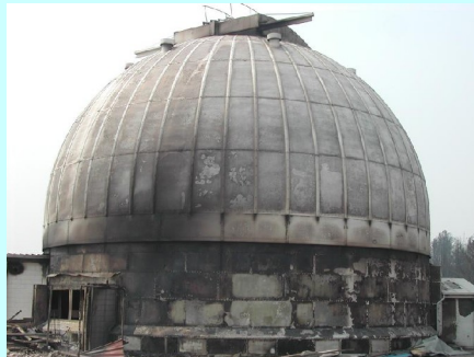
Remains of the 74 inch refractor building after the fire.
